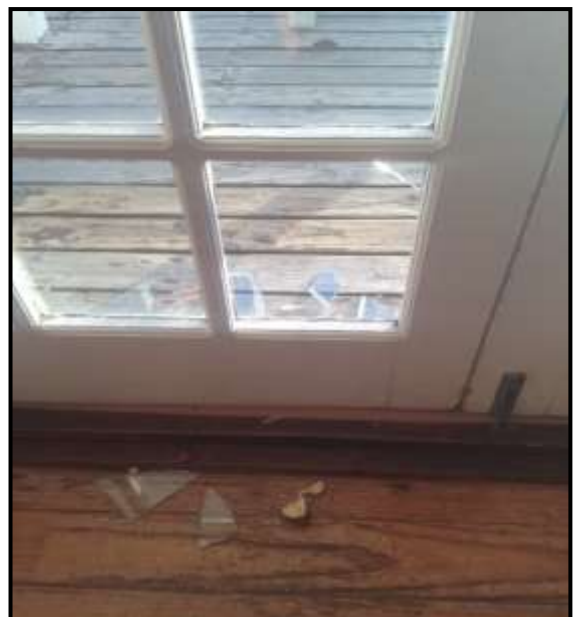
Fig. 8. Window pane broken by GOB8 in Klip St, Scarborough – April 2014
