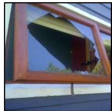
Figure 8. Window broken by GOB8 to gain access to house.
